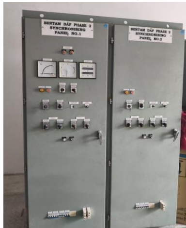
iv) Synchronising Panel
