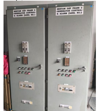
v) Generator Control & Alarm
